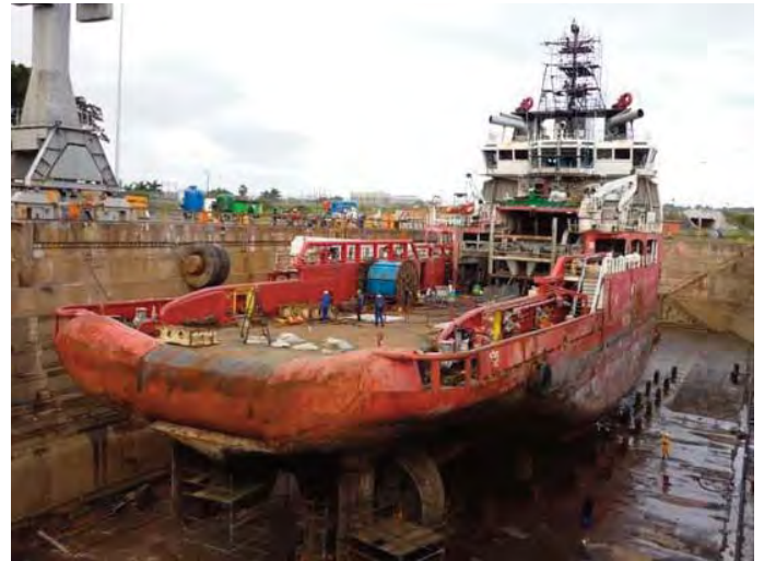
Electrical refit and full powertrain overhaul of the fire-damaged offshore tug Subhiksha, by Southern African Shipyards. A complete overhaul to the main engine and crankshaft; thrusters, propellers and main shaft. Replacement of all electrical items, including over 15km of wiring.
